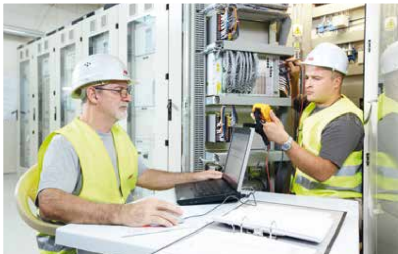
Image below: ABB engineers commission protection and monitoring equipment at a substation serving the Ras Laffan power plant in Qatar. Substation equipment provides monitoring and control functions in transmission and distribution grids, ensuring the reliability of power supplies.
